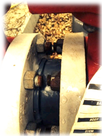
Snapped Backwash Pipe
