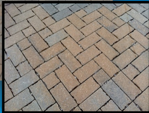
Clark Montessori High School Pervious Paver Driveway Leaf litter present, coarse sand missing May 2013
