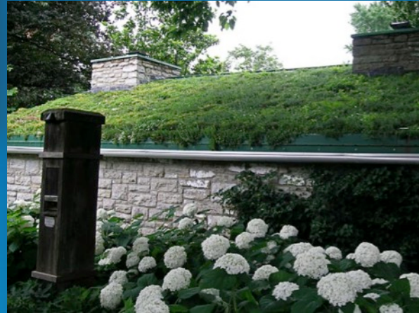
Civic Garden Center Sloped Green Roof Good condition June 2013 Civic Garden Center Photo
