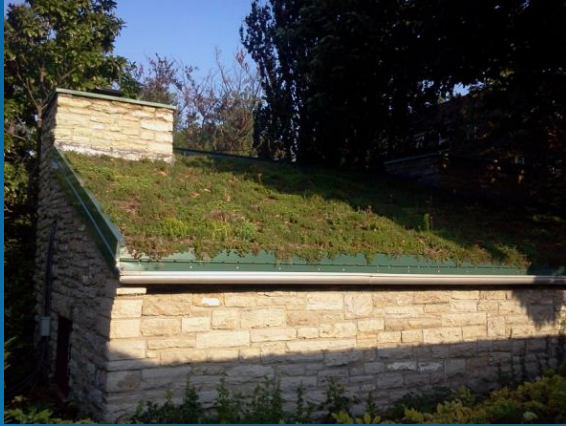
Civic Garden Center, Cincinnati, OH Sloped Green Roof – Mat Type August 2010 T. Ellwood photo
