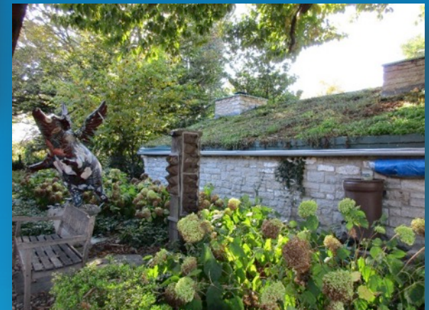
Civic Garden Center Sloped Green Roof Good condition after dry spell and freeze October 19, 2015 K. Couch photo
