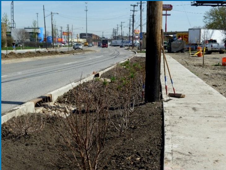
Spring Grove Avenue, Cincinnati, Ohio Bioswale after Construction March 21, 2010 CDM Smith photo
