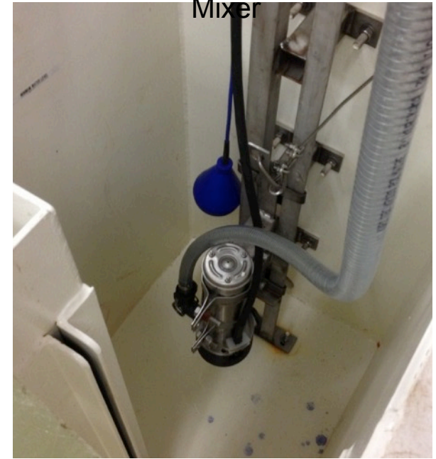
Sodium Hypochlorite Induction Mixer
