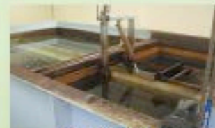
Drinking Water Treatment Plant
