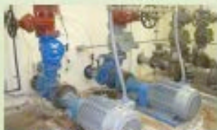
Booster Stations and Other Pumps
