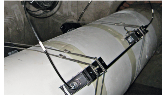
Courtesy of Siemens
