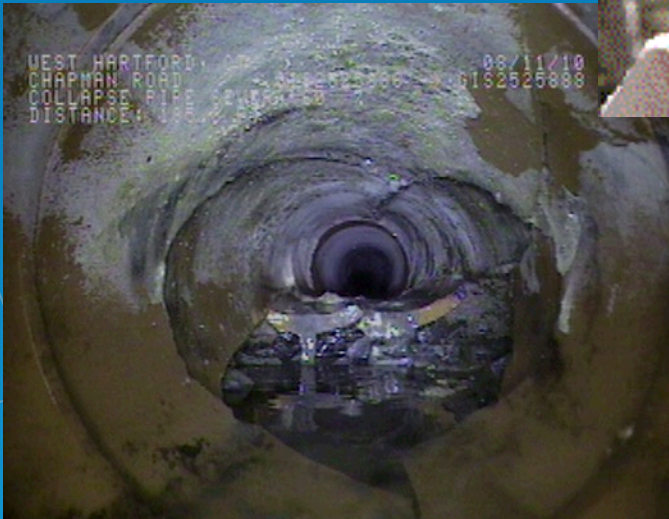
Sewer Main Defect
