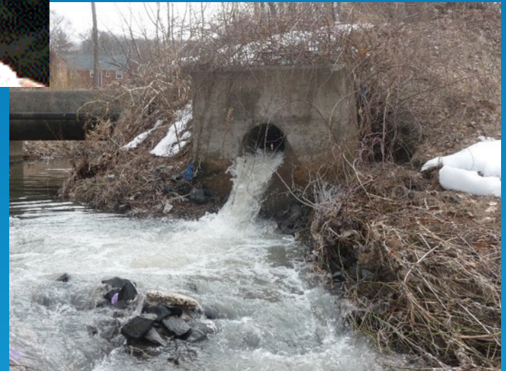
Sanitary Sewer Overflow
