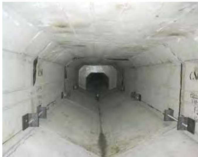
Storage conduit sections with v-notched invert
