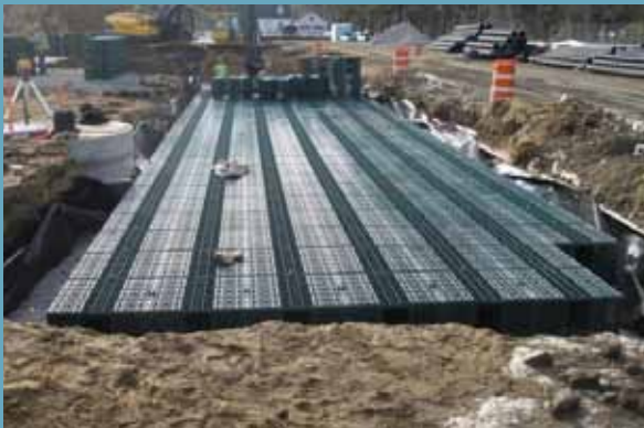
Harriet Beecher Stowe School, Brunswick, ME – Underground Detention System
