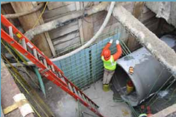
Reserved Channel Sewer Separation Project, Boston, MA – Construction of New Drain Manhole
