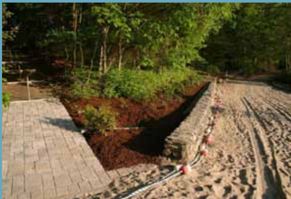
Sherborn Farm Pond, Sherborn, MA – Permeable Pavers, Rain Garden and Groundwater Recharge
