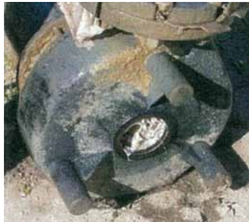
A Portland Water District (Maine) pump, clogged with wipes—an occurrence repeated across the country
