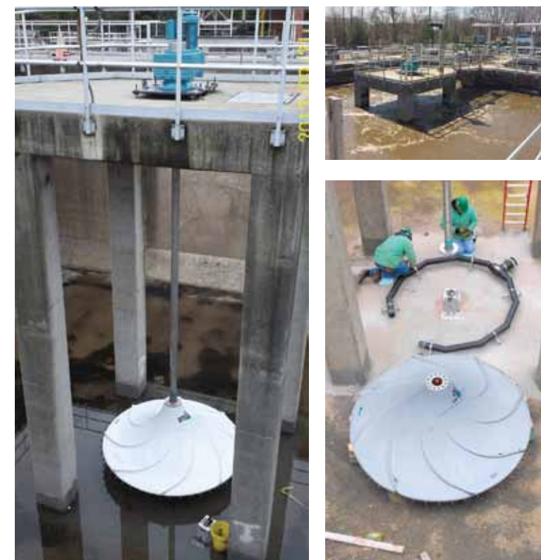
Figure 3. Hyperbolic mixer-aerator being installed and operational (top right)
